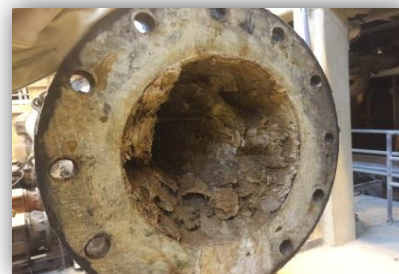
Struvite buildup in sludge piping system
