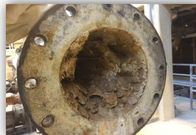
Struvite buildup in sludge piping system
